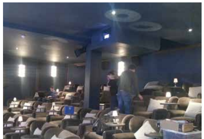
Projector housing unit mounted into the ceiling
